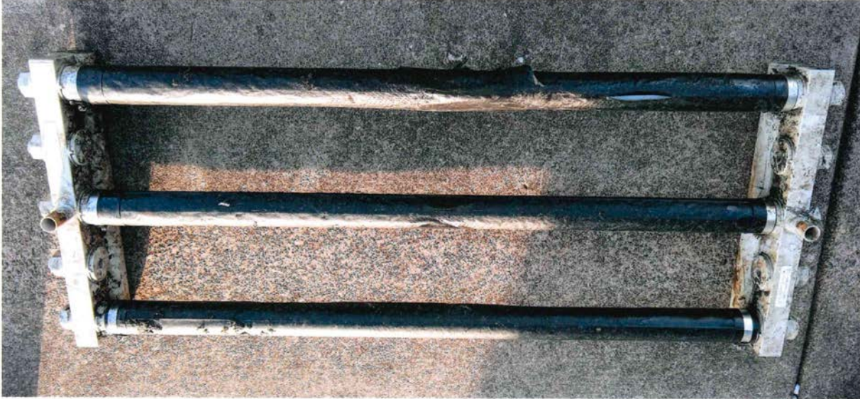
Picture of Diffuser that's suspended in the water and oxygenates the lagoons
