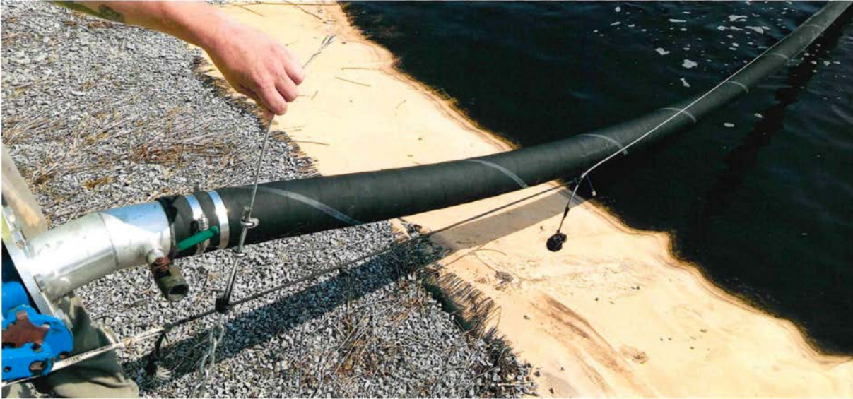
Broken support cable, Lagoon 1 Air Supply Line
