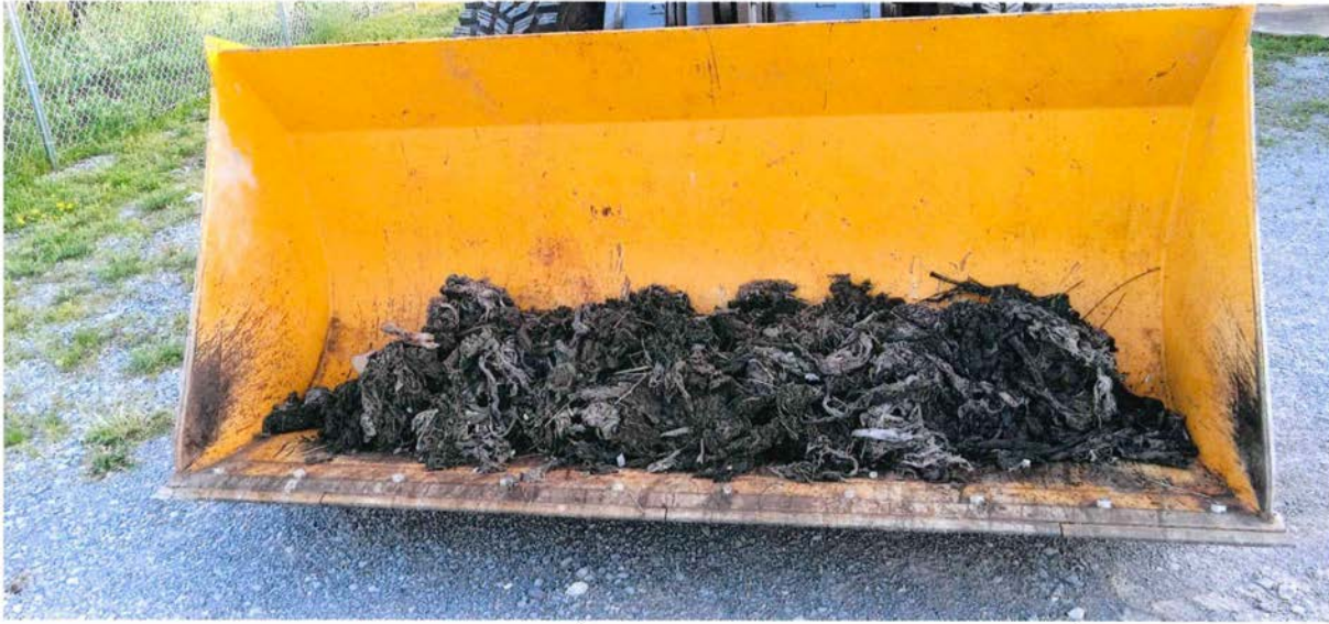
Debris removed from Diffusers in Lagoon 1
