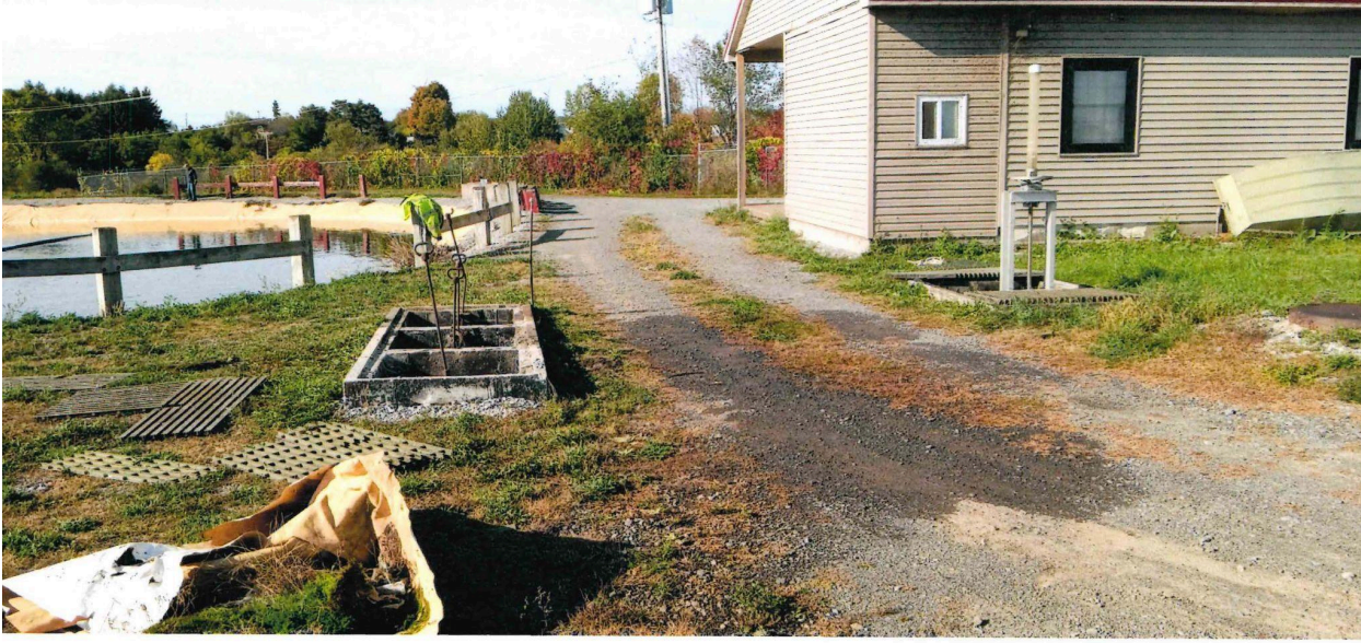
Effluent Chamber Unplugged
