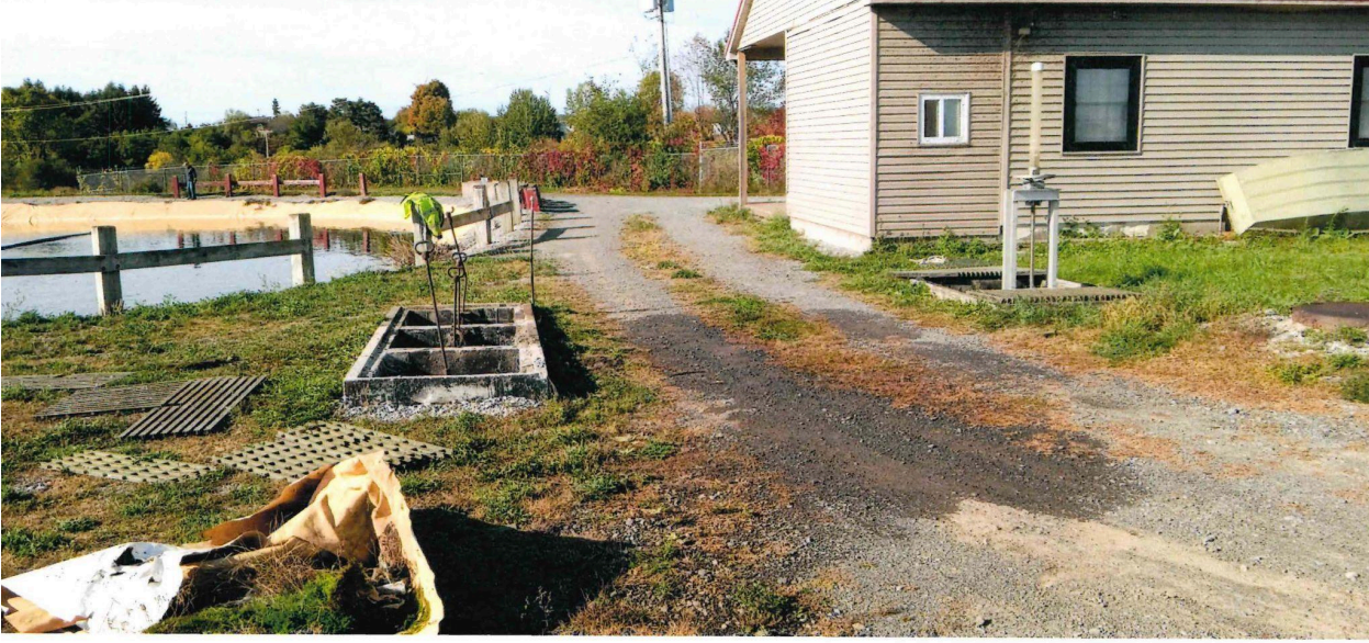
Effluent Chamber Unplugged
