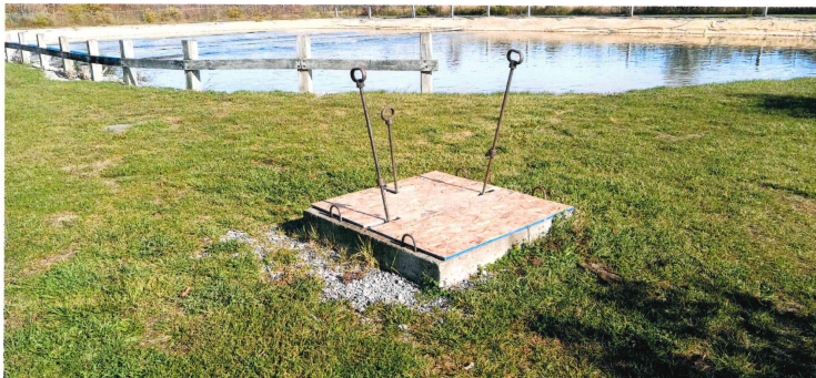
S.T.P. Secondary Flow Control Chamber Covered
