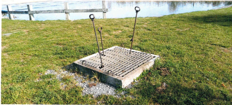
S.T.P. Secondary Flow Control Chamber Open Grid
