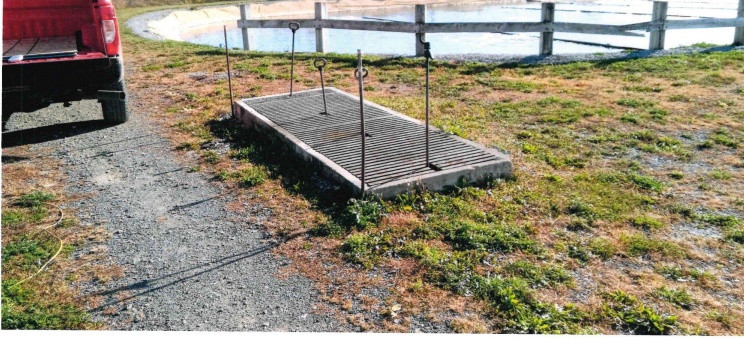
S.T.P. Main Flow Control Chamber Open Grid
