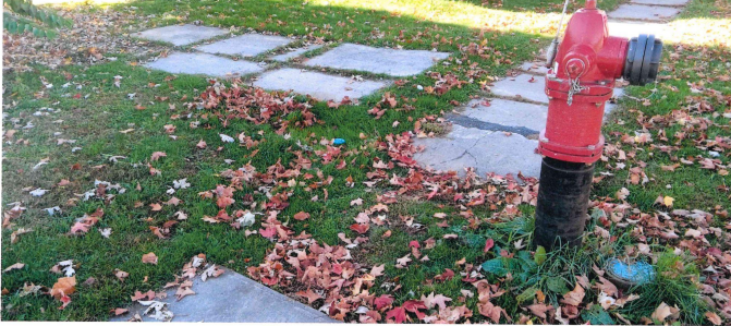
Curb Stop Required 2970 Cataract Street, Brantford
