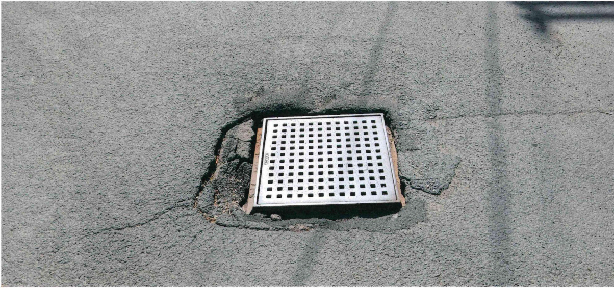
G-3-2026 Storm Drain Collapse Loud Street
